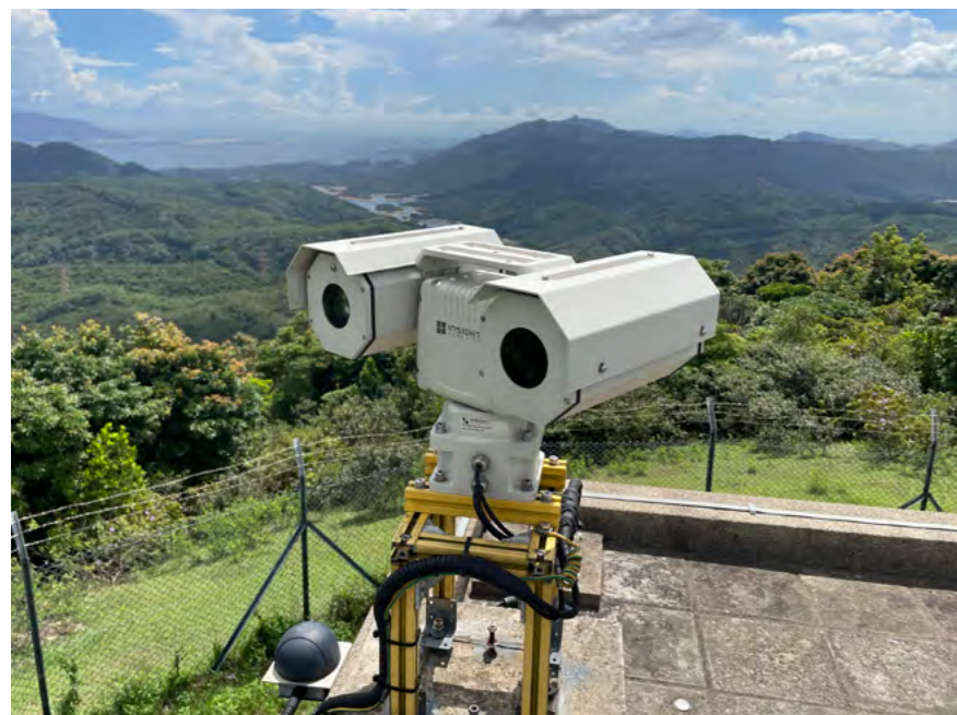
Smart hill fire surveillance system at country parks
